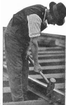
When nut breaks off it will probably hit workman on shin.
