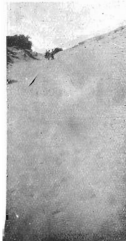
"Snap" taken by Repairer D.C. Pierce, of Sand Cutting on No. 15 Length, Nyarrin. "Yet they say sand will not drift in the winter," says Mr. Pierce. Note part of rail showing.
