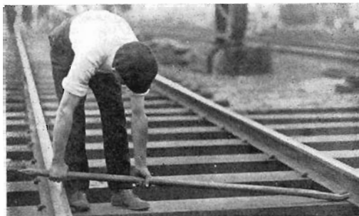
Wrong method of holding claw bar when pulling out dog spikes. Note the danger of fingers being crushed between bar and rail.
