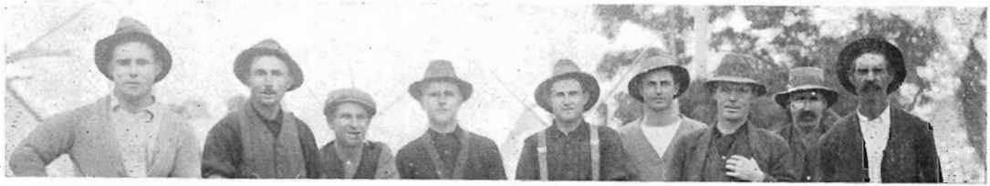
Some of the men who are repairing the track along which the Geelong Flier runs.
